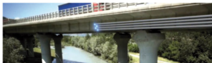
HVDC power cables installed in highway infrastructure in the future Piedmont-Savoy intertie
